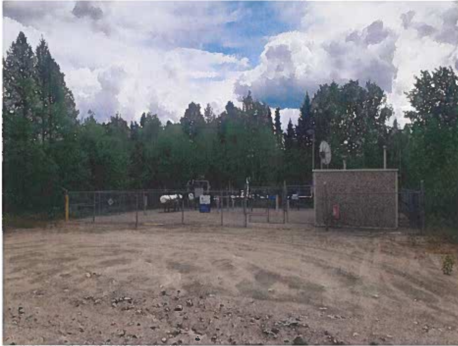
TC Energy/Union Gas/Enbridge natural gas line valve north of Ignace
